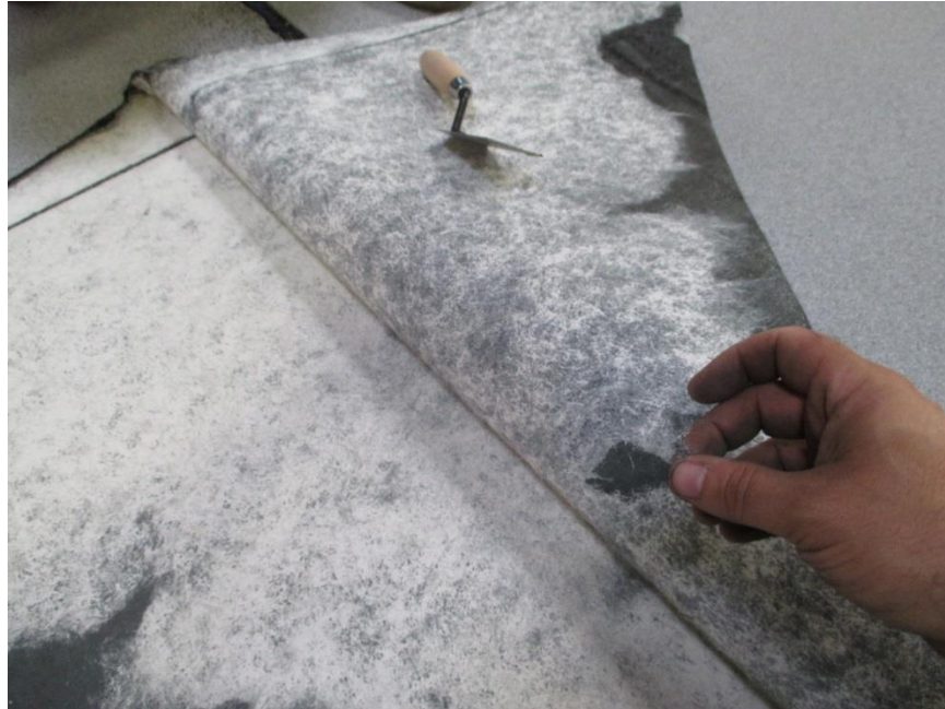
Photo No. 1 Failure Method – Facer Delamination of Gypsum Board
