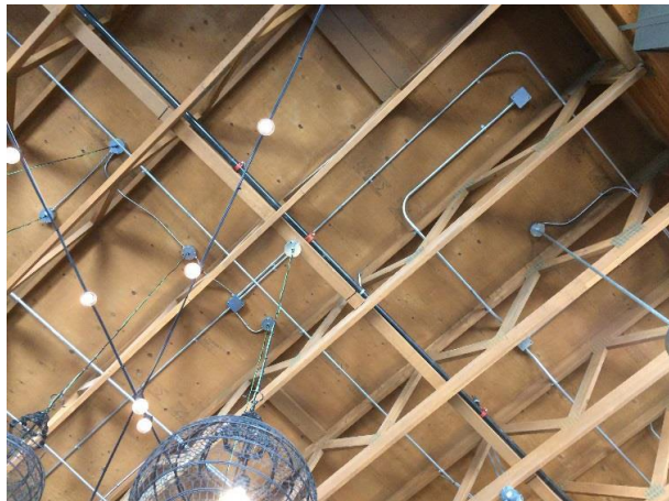
Figure 6: Junction boxes and conduit installed directly to the underside of a plywood roof deck. (Photograph by the author)
